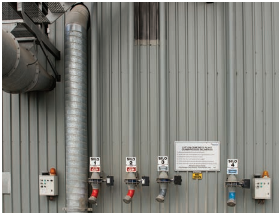
Silo delivery pipes.
